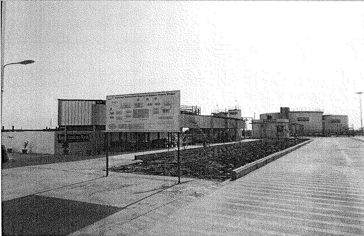
500 KLD Primary, Secondary and Tertiary Effluent treatment plant for Low Organic & Low TDS Effluent
